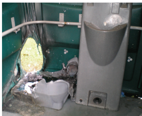
Fire damaged portable toilet in Gostrey Meadow
